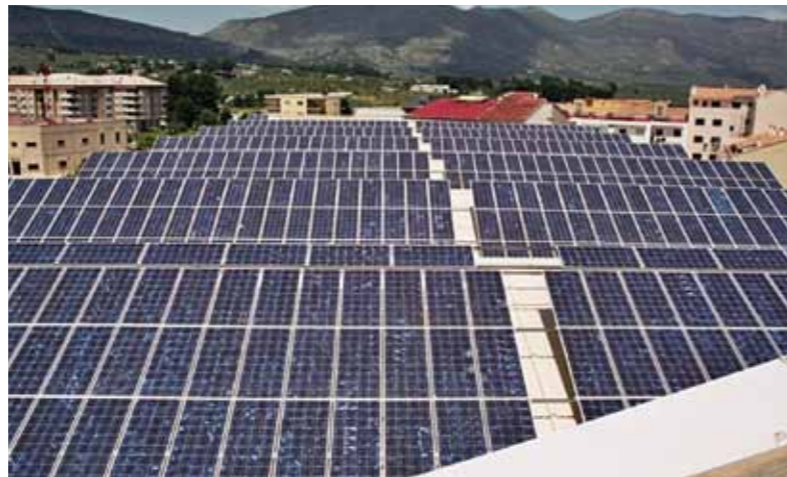
100 kWp in Muro de Alcoy (Alicante) 552 panels, 750 m 2 Annual production 157.556 kWh
