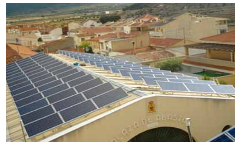
20 kWp City Hall in La Romana (Alicante) 120 panels, 160 m 2 Annual production 30.095 kWh
