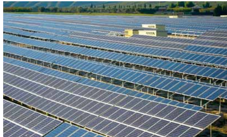
2.300 kWp in Cieza (Murcia) 10.000 panels, 150.000m 2 Annual production 3.391.683 kWh
