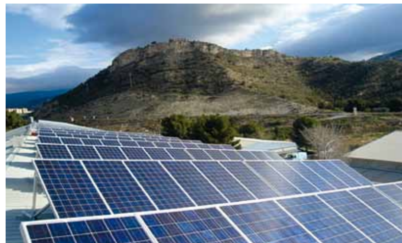
112,2 kWp in Jijona (Alicante) 660 panels, 900 m 2 Annual production 162.163 kWh
