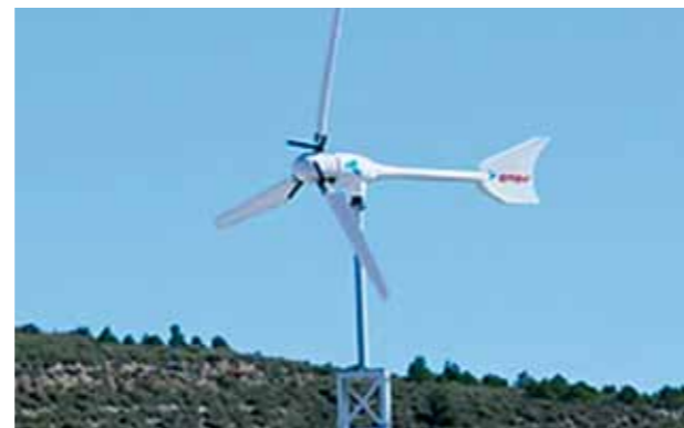
3,5 kW wind turbine in Castalla (Alicante)
