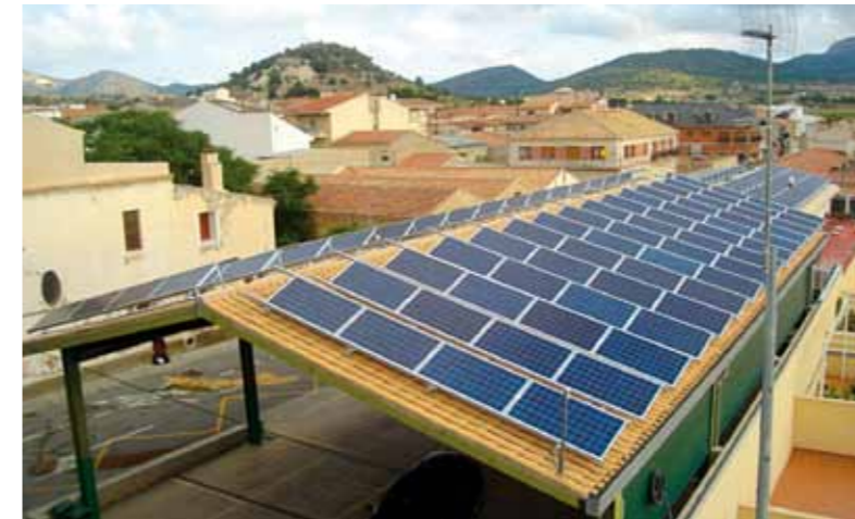
City Hall in La Romana (Alicante), 15 kWp 90 panels, 120 m 2 Annual production 22.139 kWh
