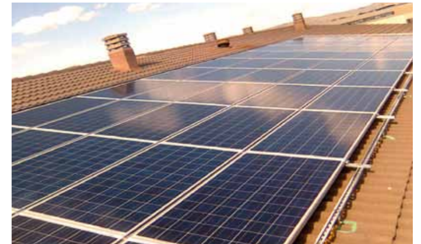
10 kW City Hall in Villena (Alicante) 66 panels, 90 m 2 Annual production 16.233 kWh
