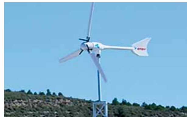
3,5 kW wind turbine in Castalla (Alicante)
