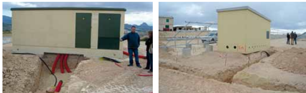
A small building is set up to protect the inverter and electrical devices from the open air.
