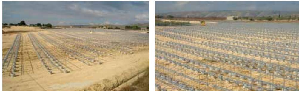
Clearing the land (around 70.000 m 2 ) and setting the metal structure for the panels.
